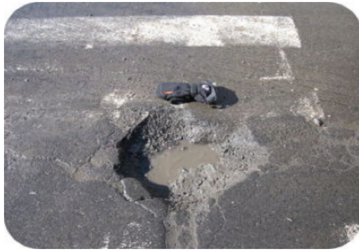
Figure 1. A once smooth road surface has cracks and fractures, plus a large pothole.
