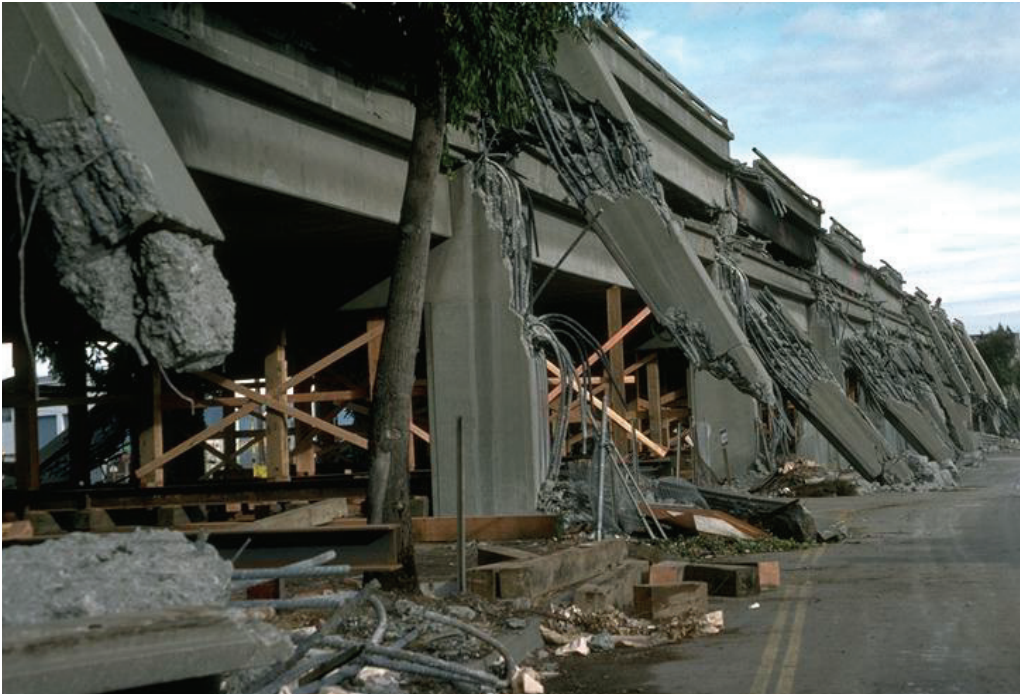
Figure 12. Structural damage due to an earthquake (Image by H.G. Wilshire, U.S. Geological Survey).
