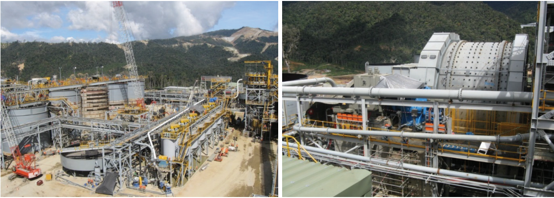
Figure 6. Crushers and ball mills used at the Hidden Valley mine, Morobe Province (Images after MMJV).
