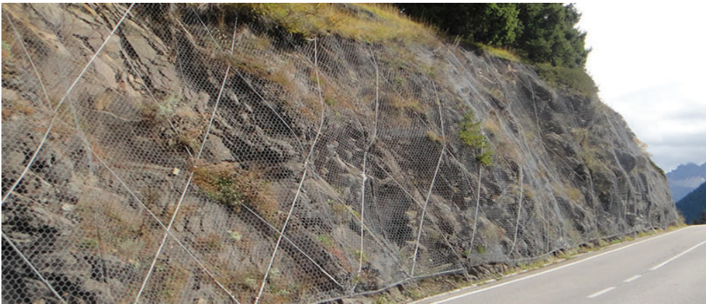
Figure 11. Rock fall netting is hexagonal wire mesh to prevent rocks from falling onto roads.
