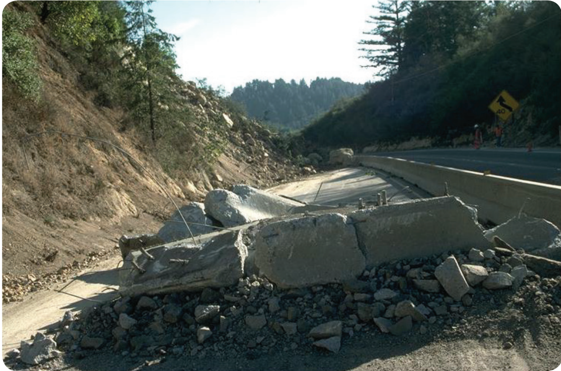
Figure 13. Debris of road damage due to an earthquake (Image by C.E. Meyer, U.S. Geological Survey)
